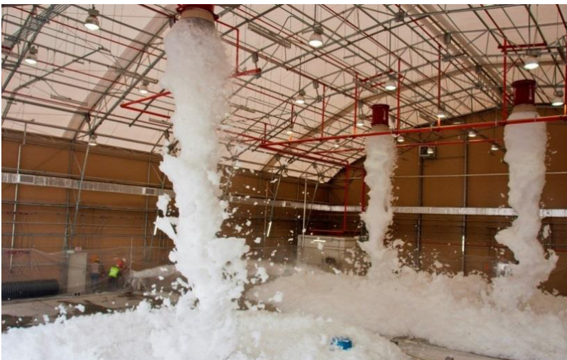
Flame retardant fills warehouse 718
