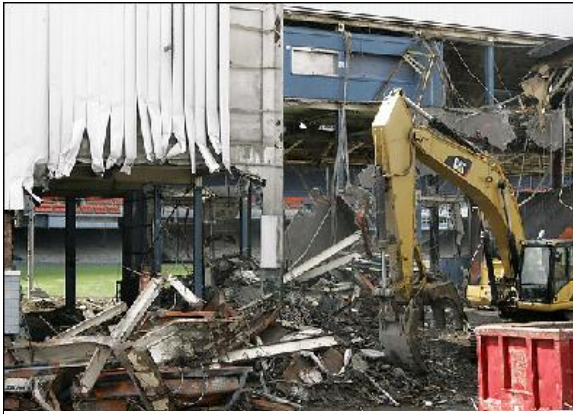
Old Tiger Stadium in need of major repairs.
